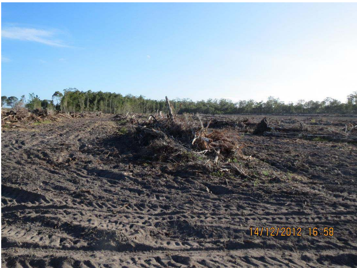
Vast area of coastal Wallum vegetation cleared (continuing) at Nolan Road Burpengary. This area of threatened coastal vegetation was offset to Ipswich region where this vegetation type does not exist.
